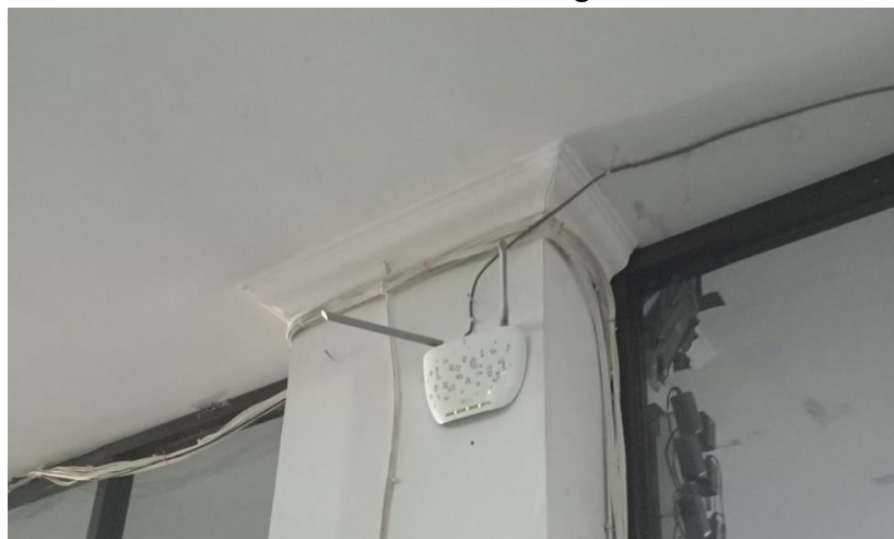
Gambar 6. Access Point lantai 1 depan
